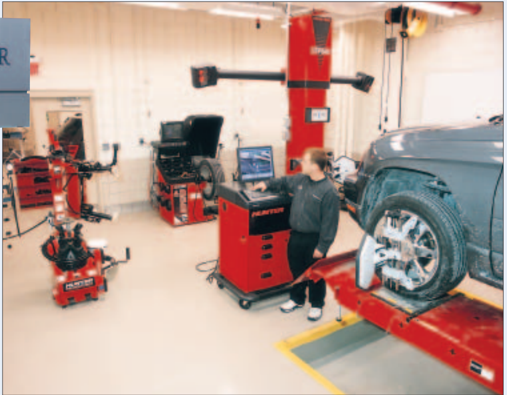
The Hunterized Wheel Service Room at DaimlerChrysler's Quality Engineering Center in Auburn Hills, Michigan.
