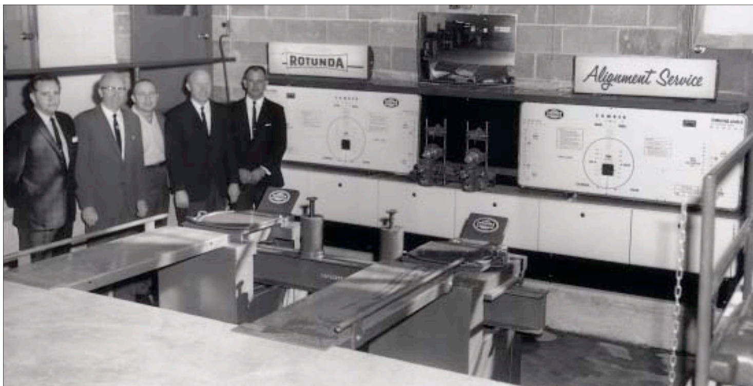
This photo shows one of the first Rotunda-branded Hunter alignment systems in a newly completed Ford service facility. The configuration is an LAD stationary cabinet with Light-A-Line instrumentation and a PE 36-in. truck pit rack. Hunter's St. Louis Regional Manager Loy Williams (far left), with Ford executives, supervised the installation.
