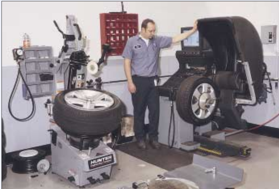
The garage renovation added this Hunter TC3500VAG premium tire changer for high-end service of specialized tires and rims.
